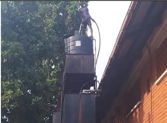
Water pressure being tested and here water was put directly to the tank.
