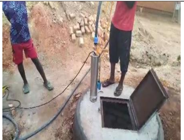
The slab is constructed and a pump installed to pump the water to the tank above
