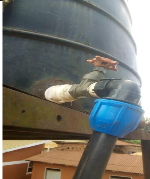
Water was connected to an existing water tank. The tank on this stand acts as the main water reservoir and distributes water to different water points by gravity
